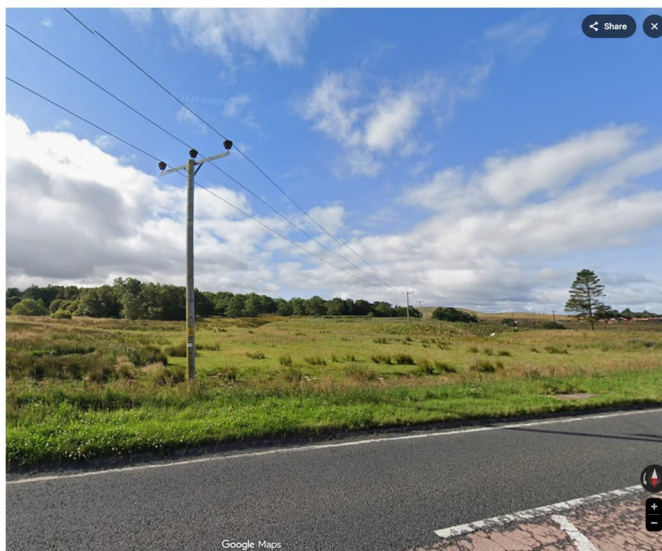
Image TA1.6.1: Image of single wood pole overhead line where it crosses over the A70 Muirkirk Road, photo facing southwest (Google Maps Streetview, accessed 15/01/2026)
