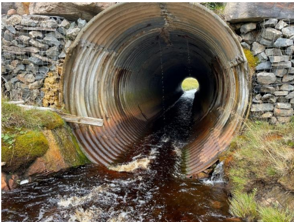
Photo 33: Gass Water - Road culvert - Partial barrier to fish migration
